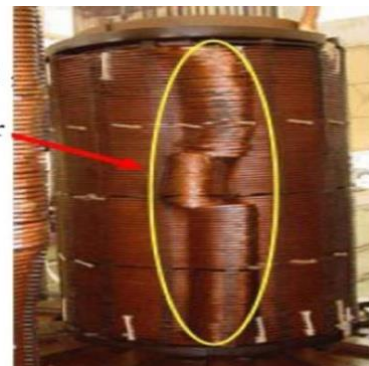
Mechanical fault of Transformer winding
