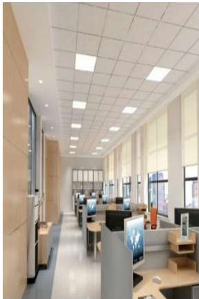
Fig 15 LED Panel Installation
